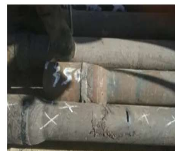
(c) Drill pipe puncture leakage[3]
